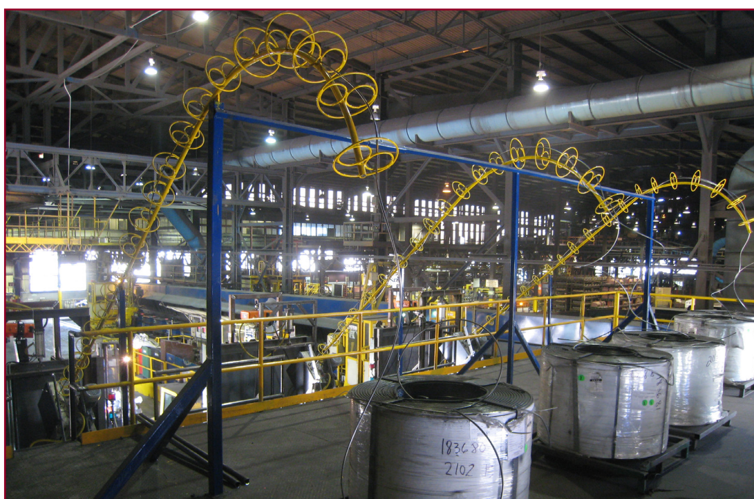
System 3000 Plus: multiple wirefeeders for base treatment and correction at the Tupy Saltillo foundry in Mexico (Courtesy, Tupy)
